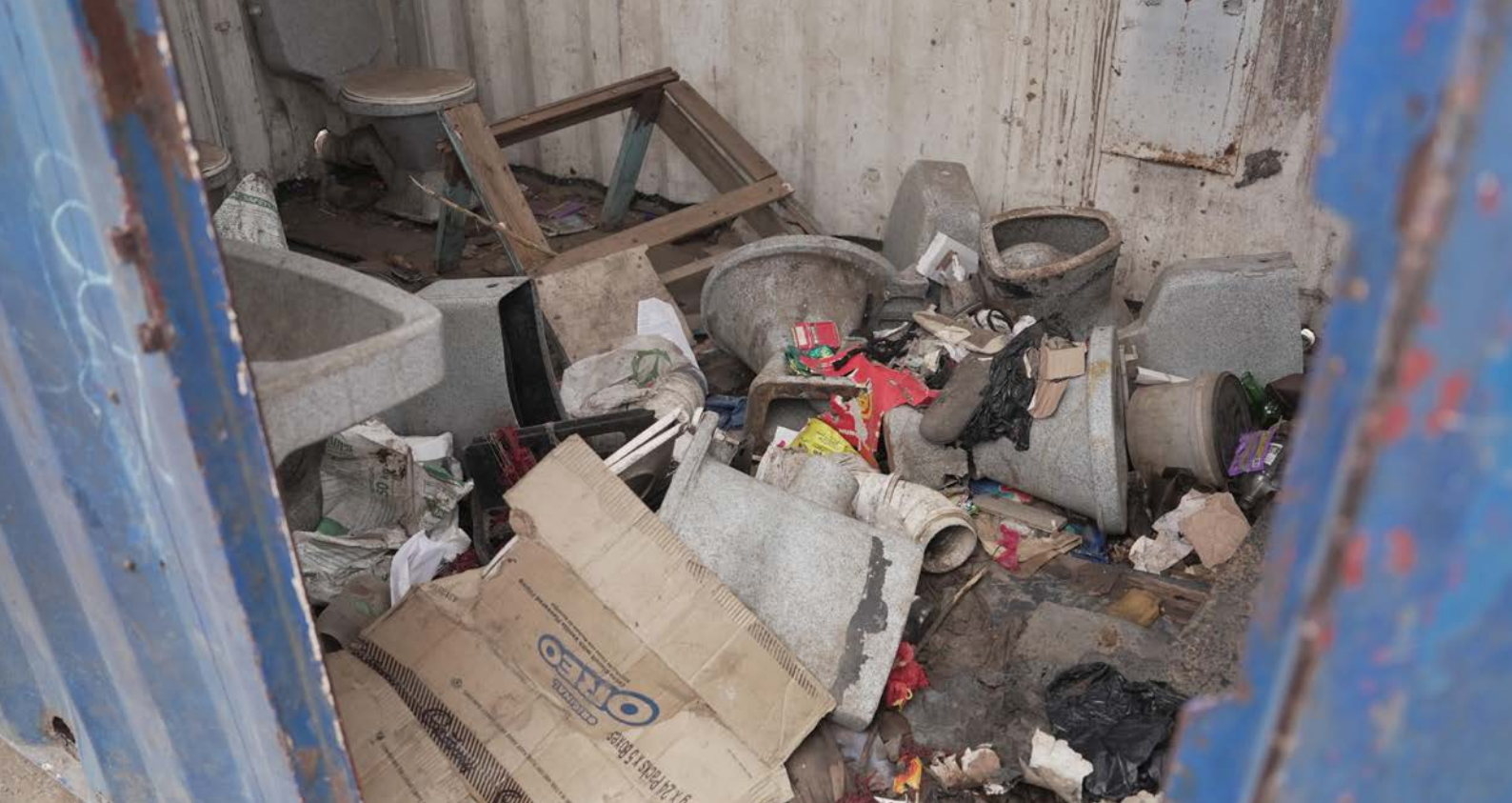
Dilapidated sanitation services in Barcelona 2 informal settlement, eThekweni, 2025 © Amnesty International
